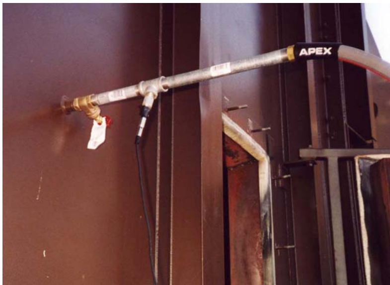
Figure 2. Example of Actual Waveguide Measurement System Installed on Gas Turbine Exhaust Duct
