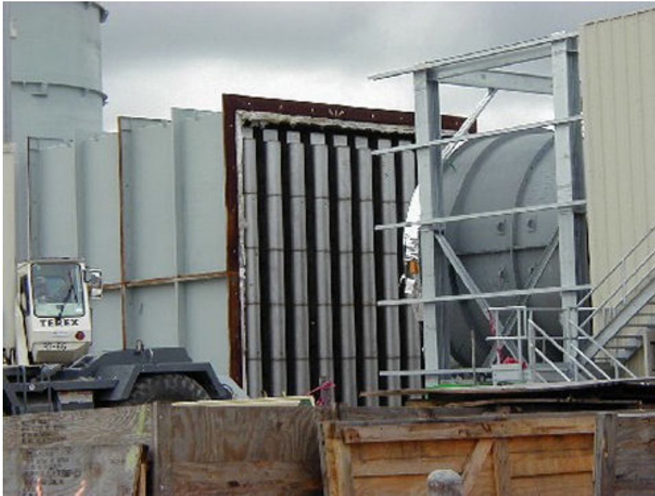
Fig. 1 – Installation of a horizontal gas turbine exhaust silencer
